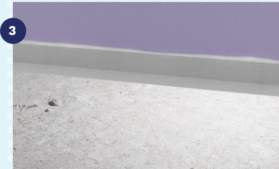
STEP 3. Bed the preformed corners and jointing tape into the wet membrane, paying particular attention to the overlaps. Ensure all air bubbles have been
