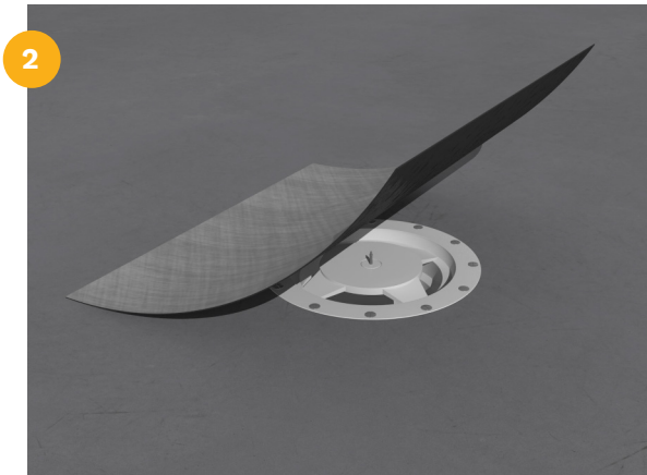
2 Mount drain seal mat centered over the floor drain with the adhesive side down and the fiber surface upwards.
