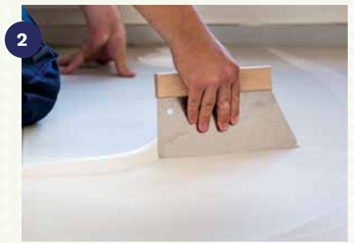
2 Pour the adhesive on the subfloor and apply the product with the spatula A2 ( \approx 260 \text{ g/m}^2 ). To ensure good transfer of the adhesive to the floor covering, observe an appropriate waiting time (5-10 min).
