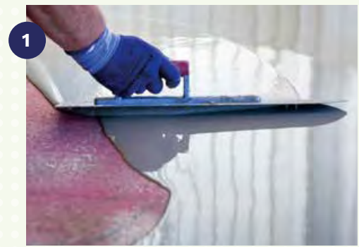
1 Prepare the subfloor with the accurate Bostik Self levelling compound associated with Bostik primer.
